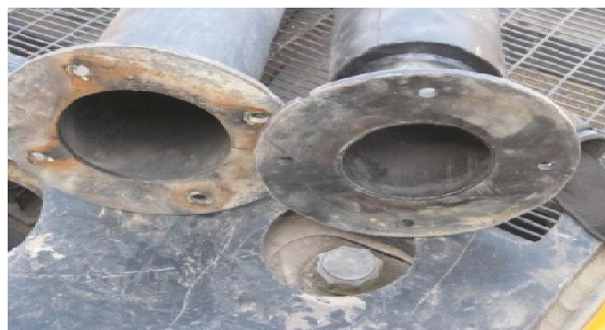
Fig. 6: Showing Silencer WLS with problems failure
